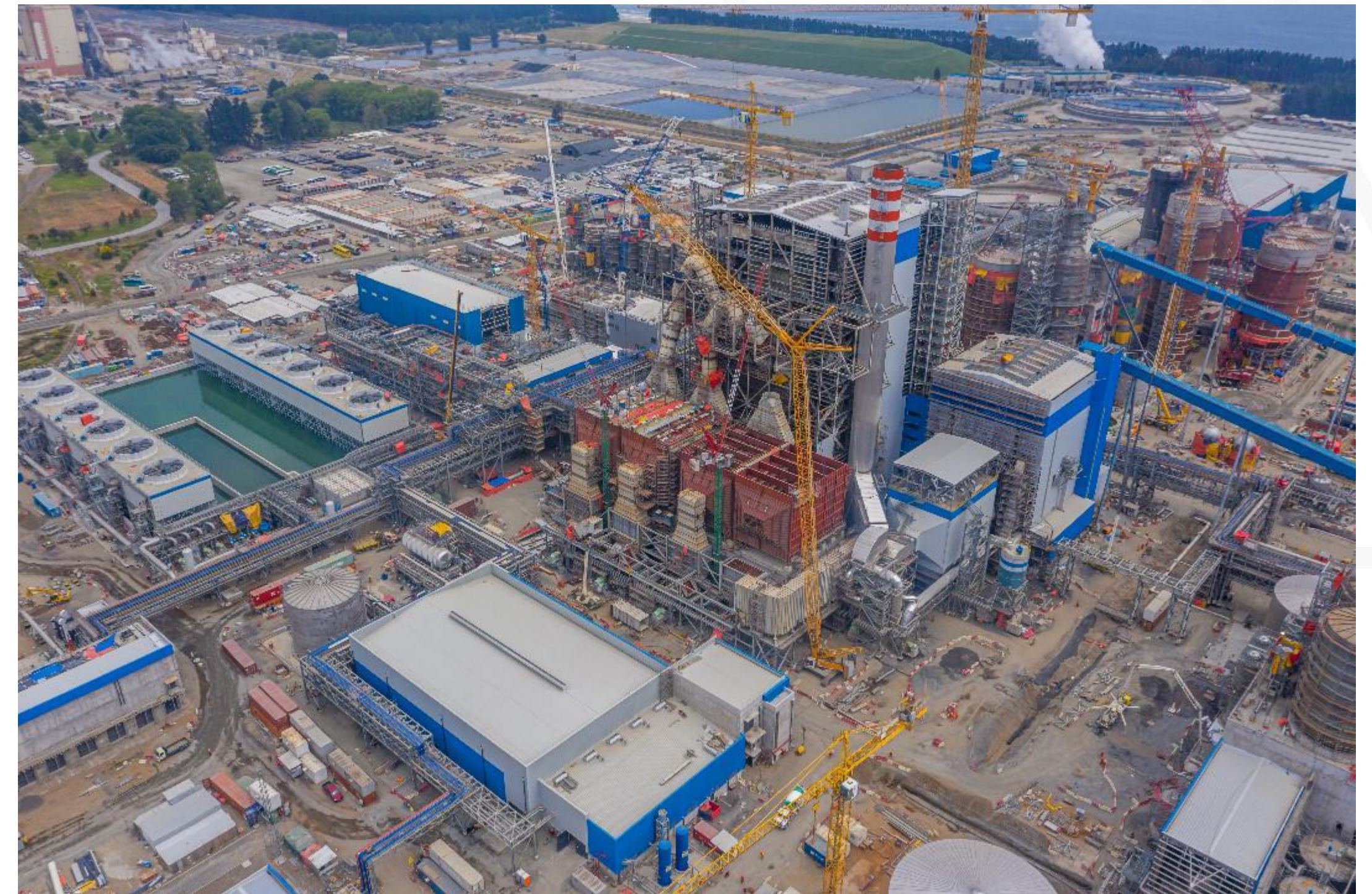
Detail (Boiler, Cooling Tower, Digesters)
