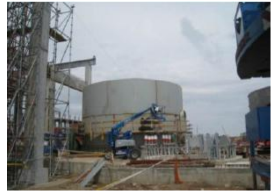
Fiberline – bleaching reactors
