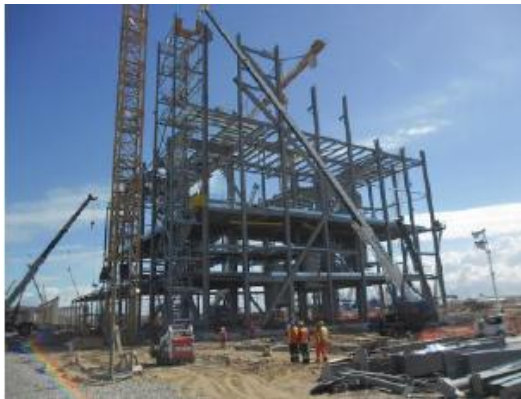
Power and recovery boiler
